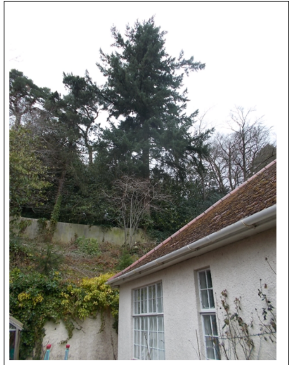
Front side and rear views of 17 Shrewsbury road the new tiles show the extent of damage to the bungalow
